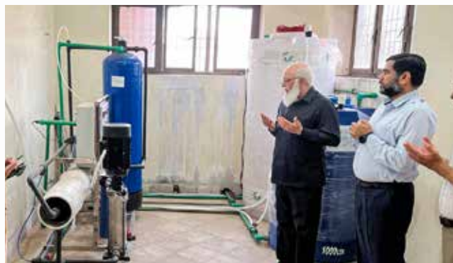
Inauguration of Water Treatment Plant
